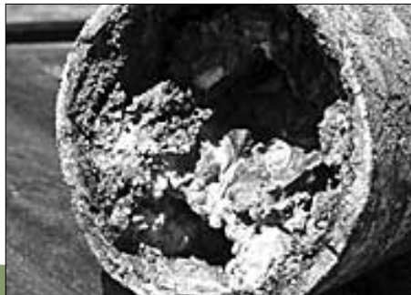
Grease in Sewer Line
